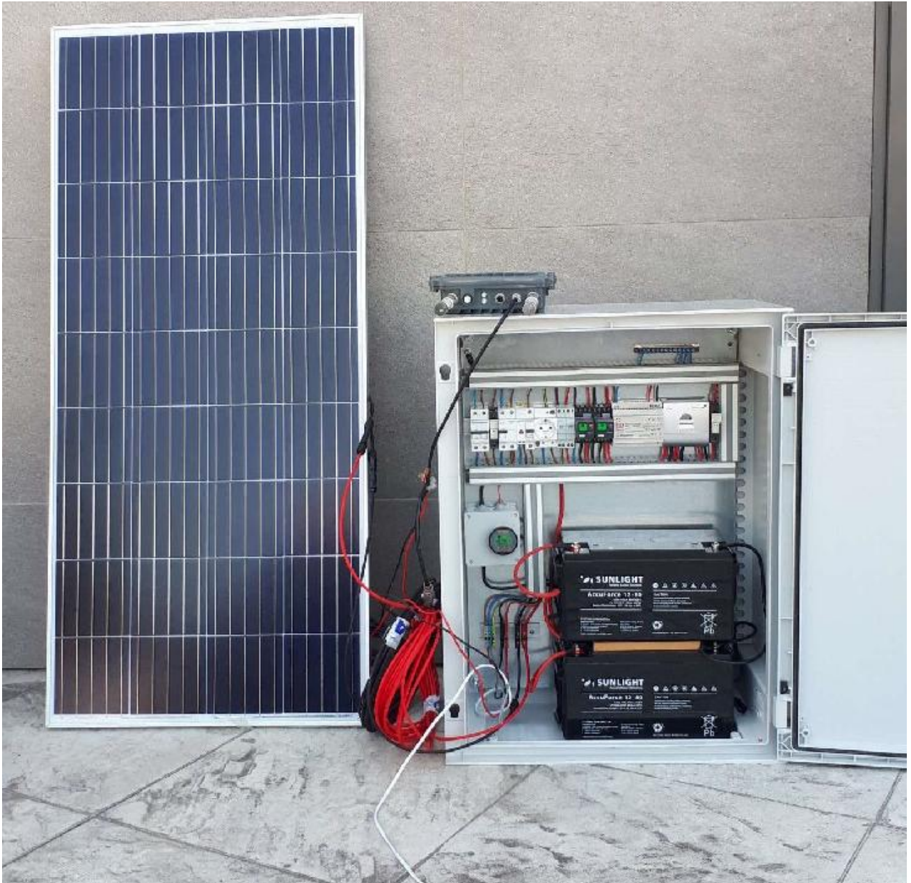
RSU Power Supply Control Panel
