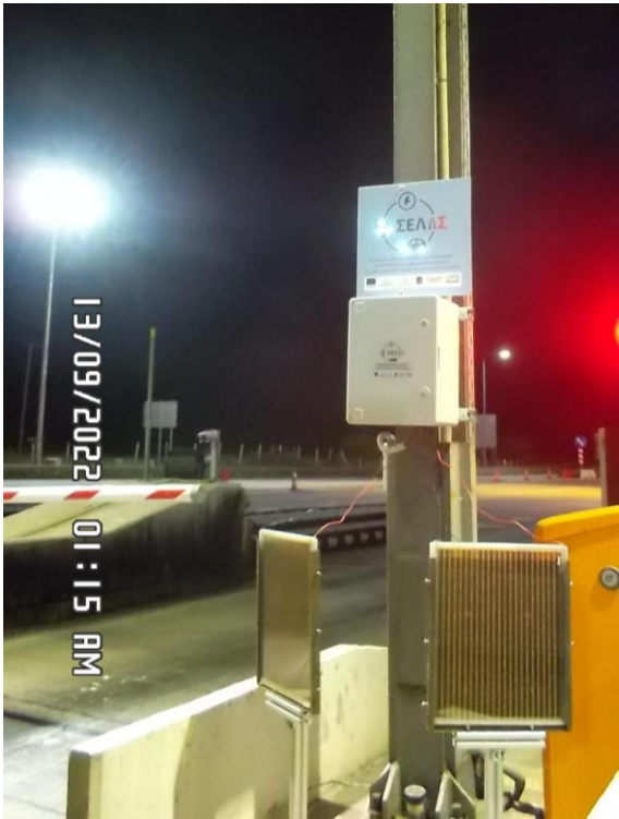
DSSC PV - Night Operation of the System
