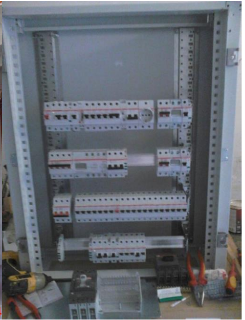
Electric Panel Building
