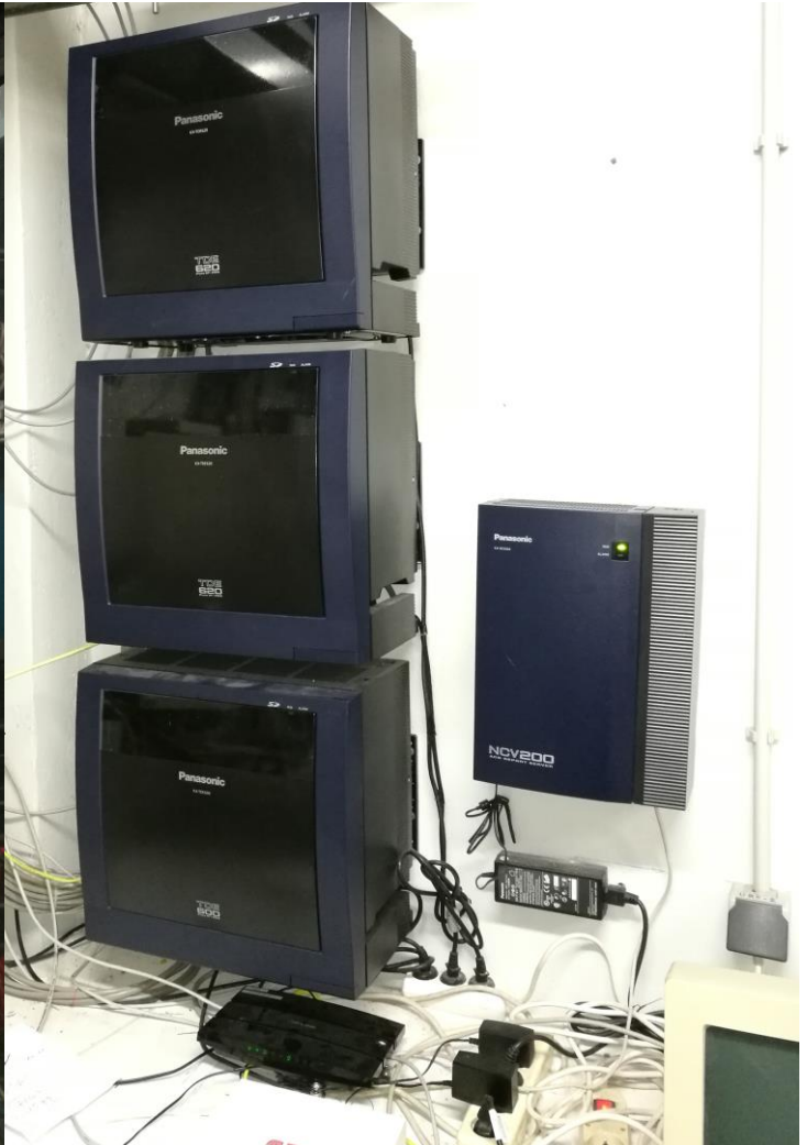
Panasonic KX-TDE600 Installation
