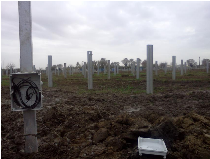
Photovoltaic Park in Arta
