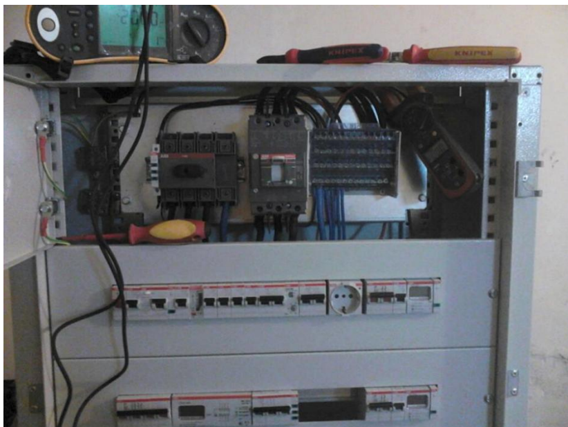
Electric Panel Inspection
