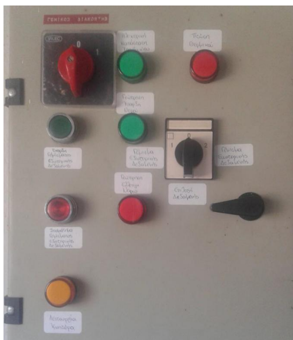
Front Panel of Automatic Water Well Control Board
