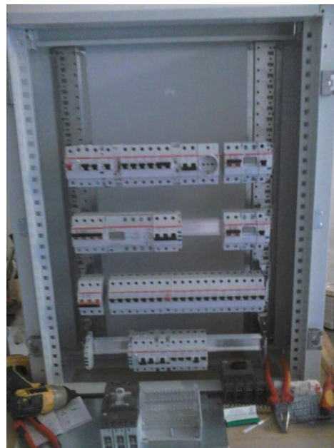
Electric Panel Building
