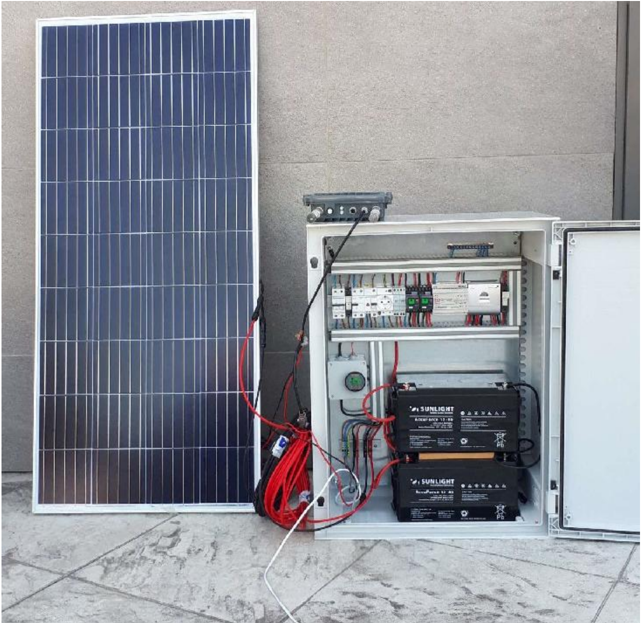
RSU Power Supply Control Panel
